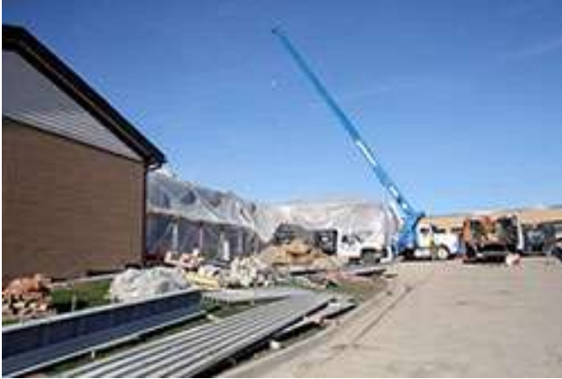
↑ New exterior and interior masonry walls go up in the south wing.
