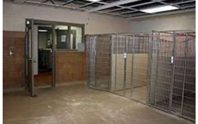
↑ With just a few minor items to complete, we are checking this phase as "Complete."
